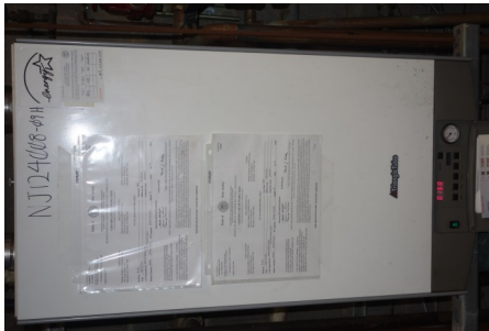
2x Triangle Tube Prestige Gas Boilers, 535000 BTU output
